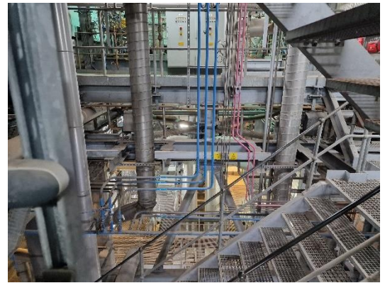
Figure 2 inside the Energy Recovery Facility
